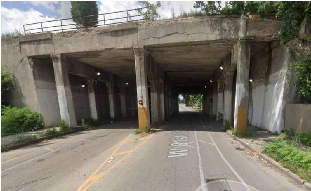
Figure 2 Deteriorating Viaduct at W. 81st St. and Wallace St.
